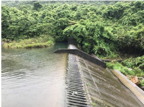
Figure 5.1: Shek Pik Reservoir Intakes
